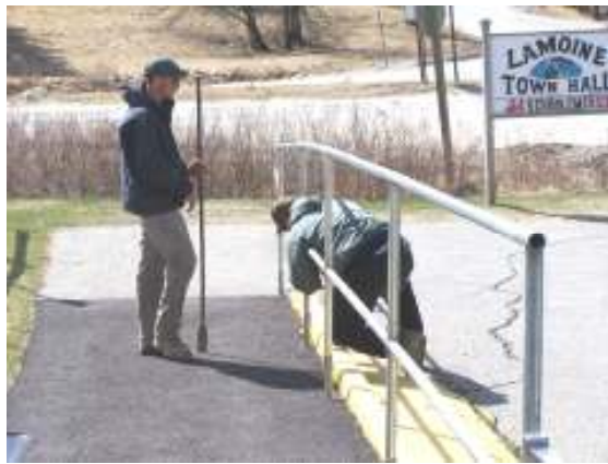
Workers from ADA Fence Company install a railing along the access ramp to the town hall.
