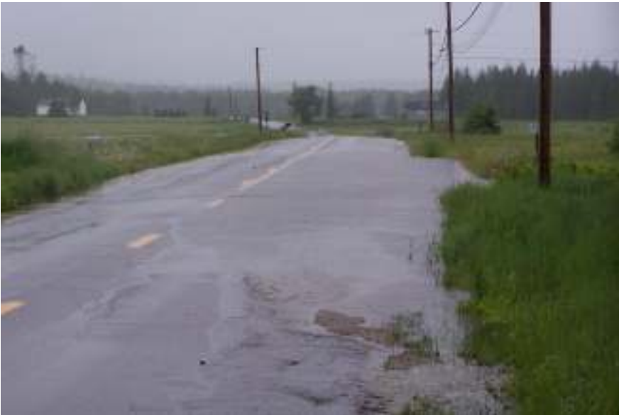
Flooded portion of Mud Creek Road
