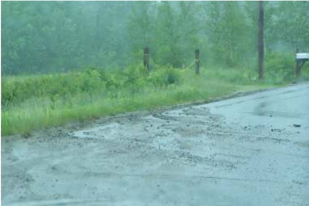
Typical shoulder washout on Buttermilk Road by Charles Gray Property
