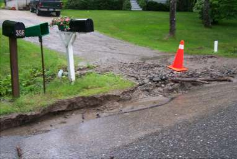
Driveway at 395 Buttermilk Road washed out.
