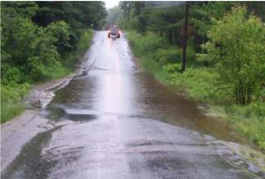
The usual flood spot on Needles Eye – this is the area for which we've submitted a Hazard mitigation grant (preliminarily approved the day before the storm!)
