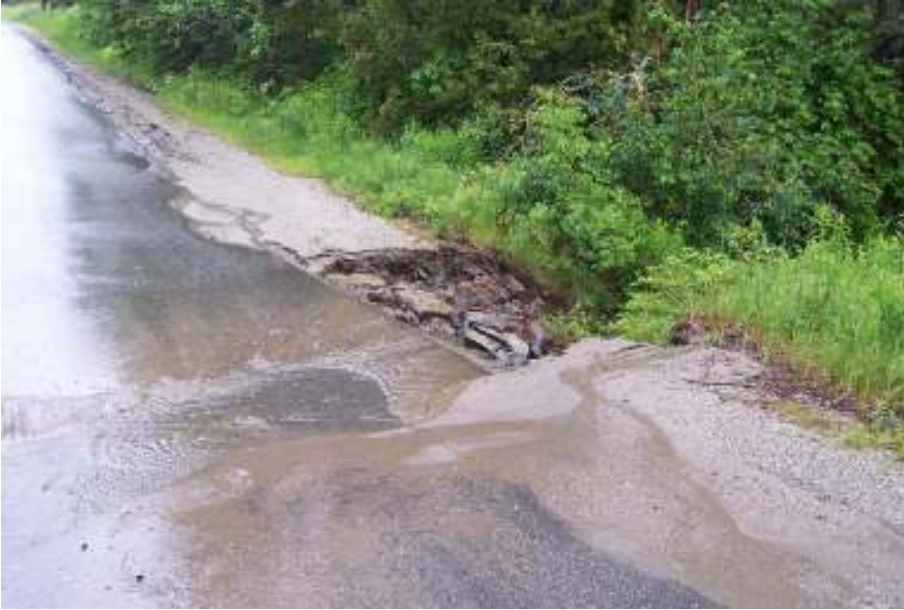
This shows the outlet of a culvert area that washed out during the storm. This is on the eastern end of the road, prior to the usual flood spot.
